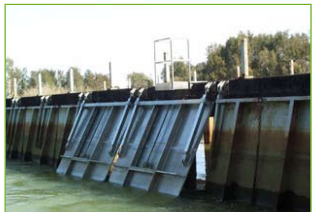
Actively managed floodgates, to allow fish passage and salt water to naturally flow upstream, source: OceanWatch Australia
