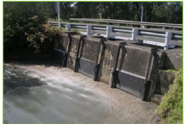
Floodgates on Crookhaven River, NSW, source: NSW DPI
