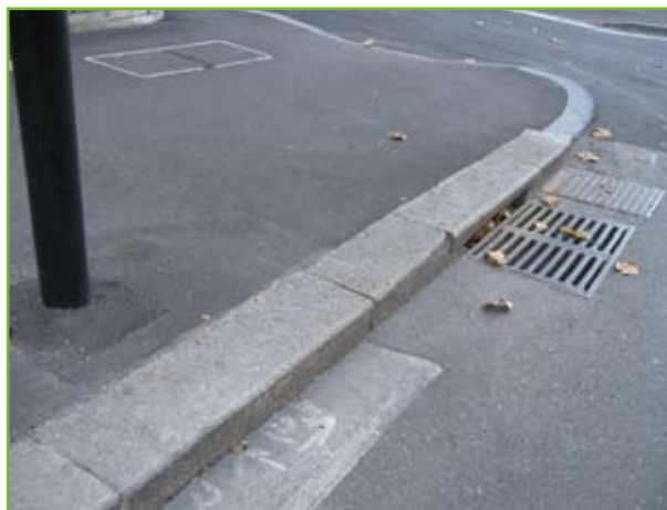
Street gutters and drains, source: OceanWatch Australia
