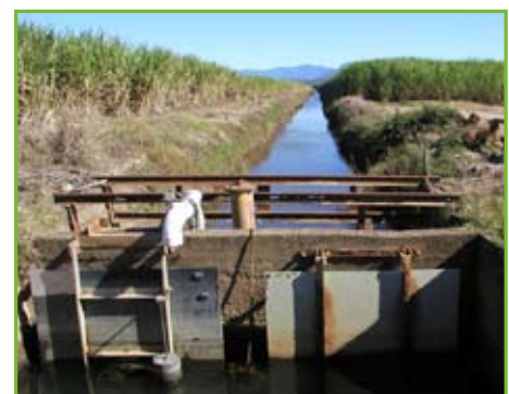
An example of floodgate structures on a drained floodplain, source: OceanWatch Australia
