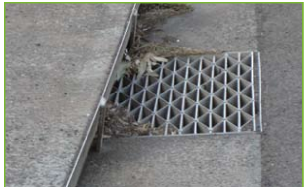
Kerb and gutters in Nowra streets, source: OceanWatch Australia
