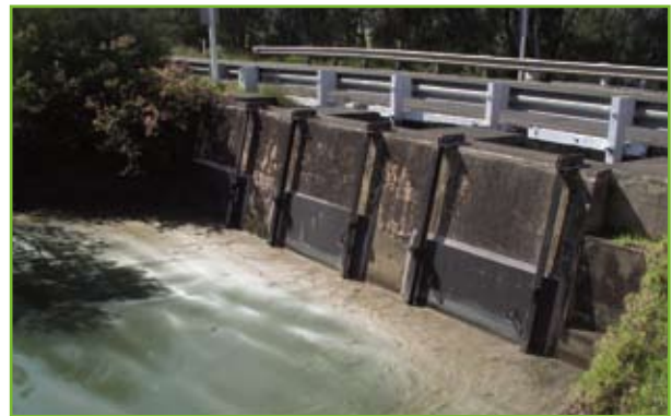
Floodgates on the Crookhaven River, source: NSW DPI (Scott Nichols)
