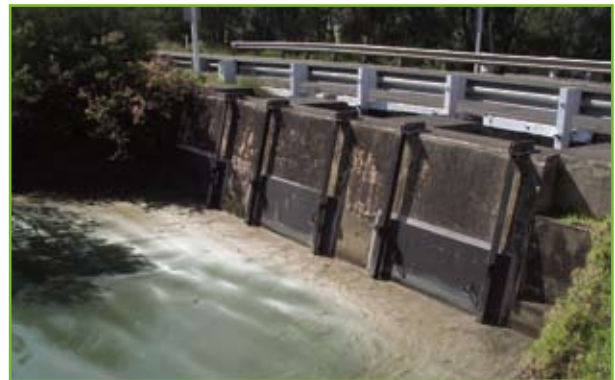
Floodgates on the Crookhaven River, source: NSW DPI (Scott Nicols)
