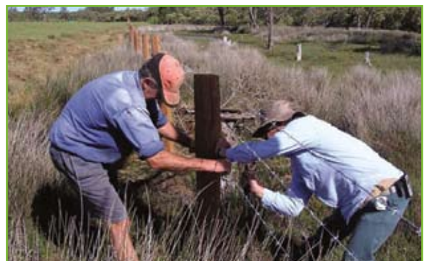
Greencorps team helping landowners fence cattle out of the Shoalhaven River, source: SRCMA
