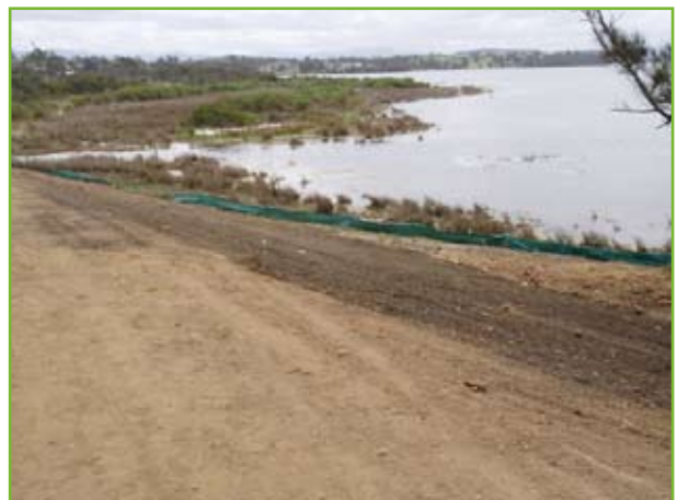
Removal of vegetation cover exposing soil to erosion, South Coast NSW, source: OceanWatch Australia
