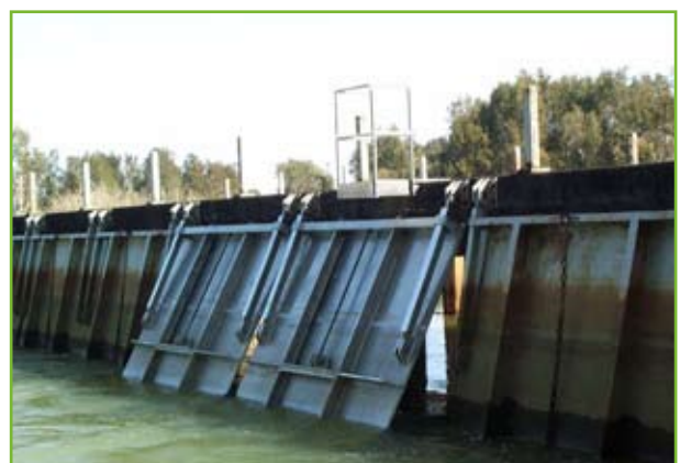
Actively managed floodgates, to allow fish passage and salt water to naturally flow upstream, source: OceanWatch Australia
