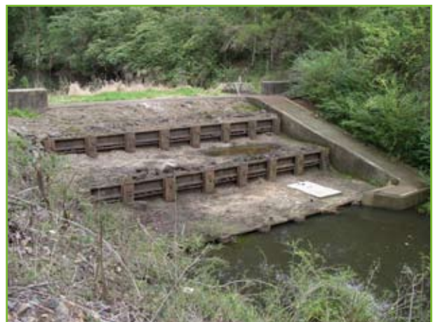
Weir on Ourimbah Creek, Central Coast NSW, source: NSW DPI/Wyong Shire Council
