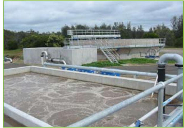
Sewage treatment plant, source: Bega Valley Shire Council
