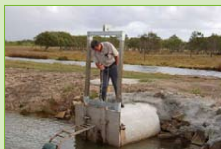
A tidal floodgate with a winch which allows for improved water exchange, source: Clarence Valley Council
